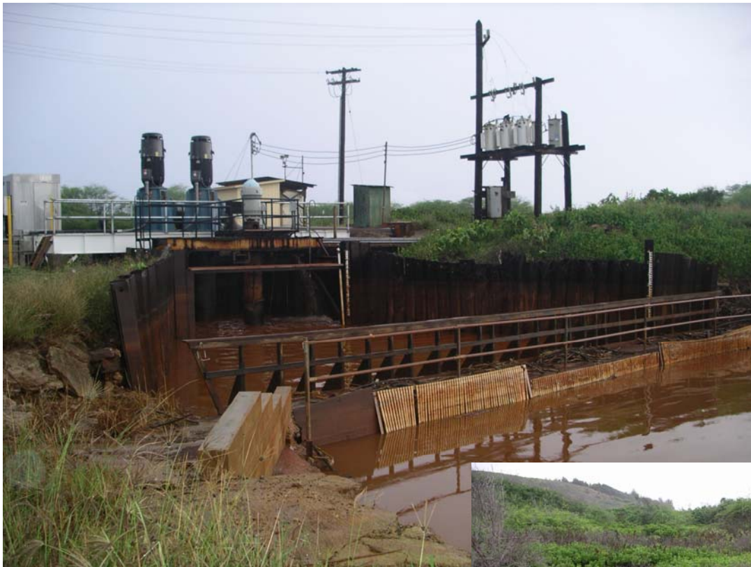
Kawaiete Pumping Station, Mānā Plain, Kaua'i
